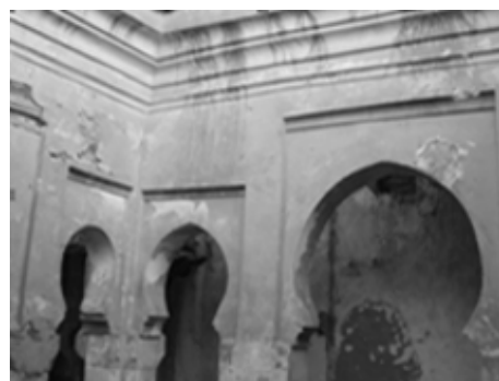
Figure 19. Cracks and degradations of earthen arches: The absence of the protection of the roof caused cracks, excavations and erosion of the earth material at the level of the bearing structure of the house in particular at the level of the arcades. Source: Authors.
