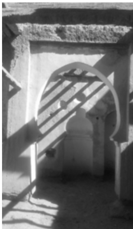
Figure 17. Cracks and degradations of earthen arches: The absence of the protection of the roof caused cracks, excavations and erosion of the earth material at the level of the bearing structure of the house in particular at the level of the arcades. Source: Authors.
